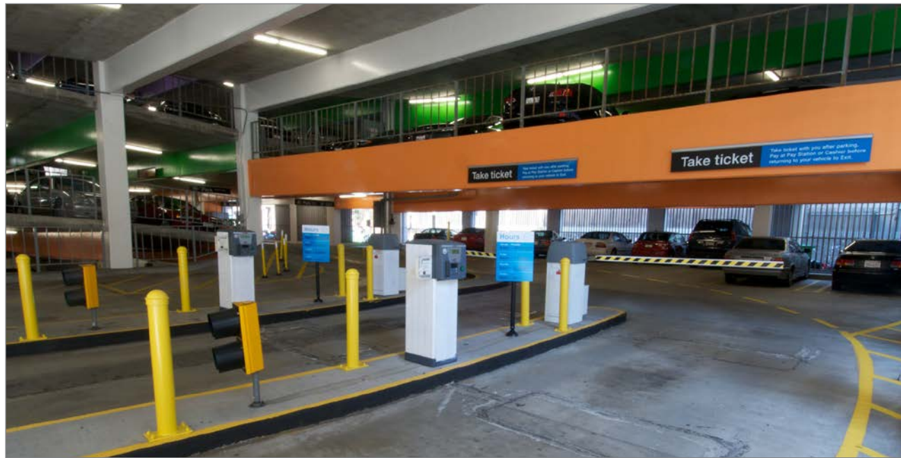
The entry and data collection system at an SFpark garage ▲
