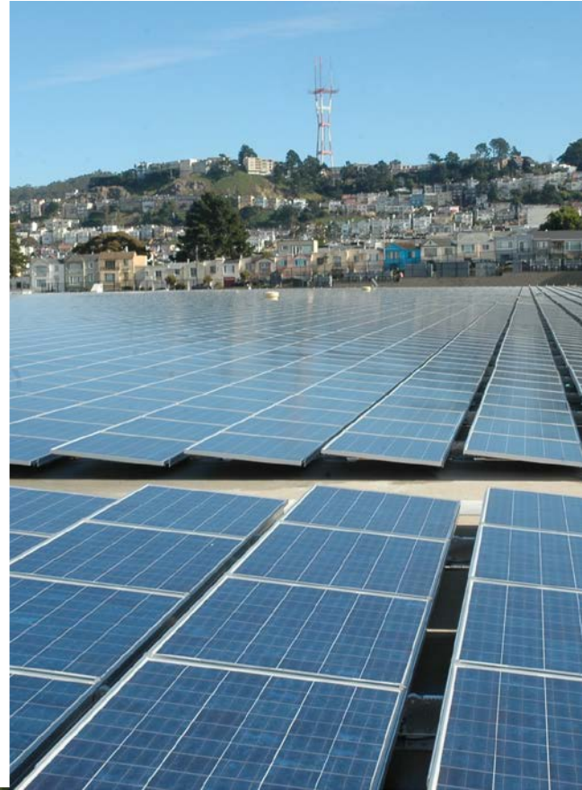
Solar Panels at Sunset Reservoir
