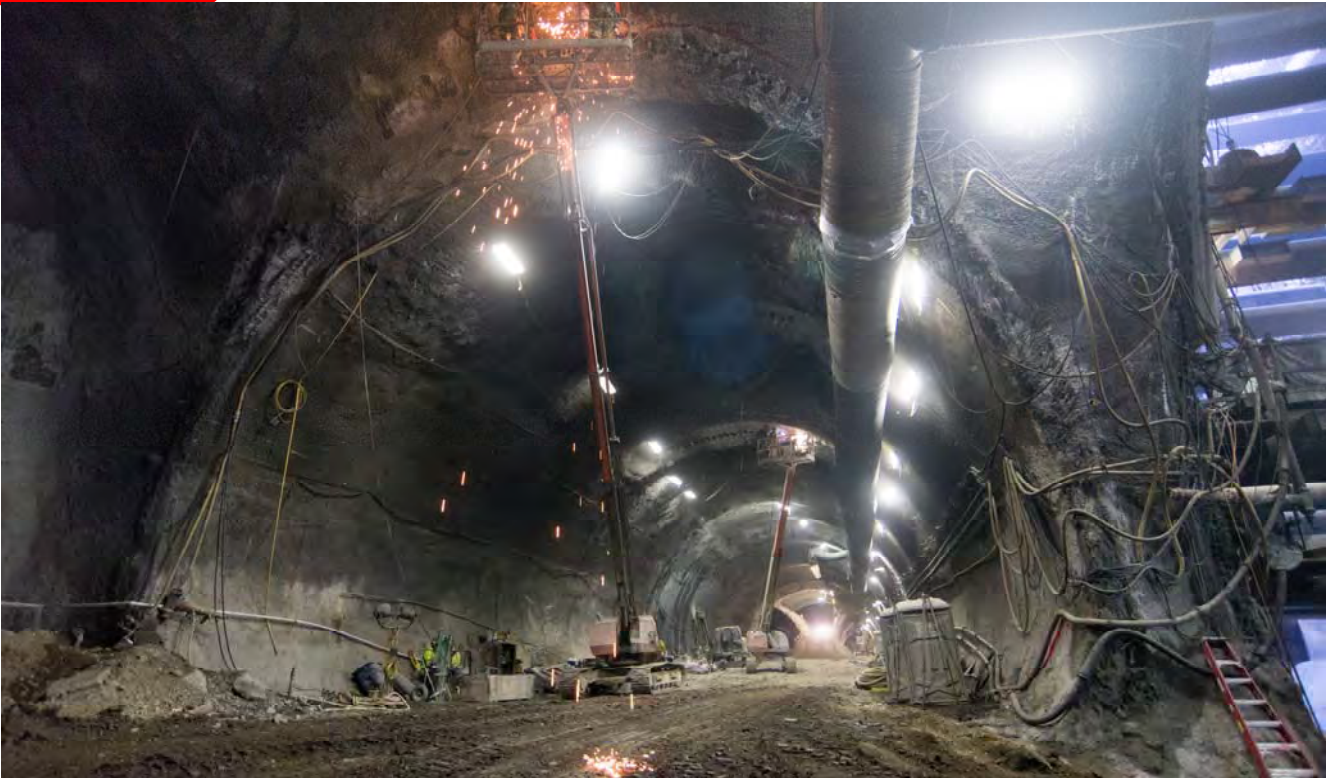
Sparks fall from a man basket where two workers cut away exposed drill casing segments in the massive arched structure of the platform cavern.
