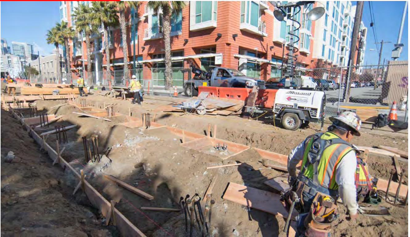
Concrete forms are being constructed to build pile caps for the 4th and Brannan surface station platform foundation.
