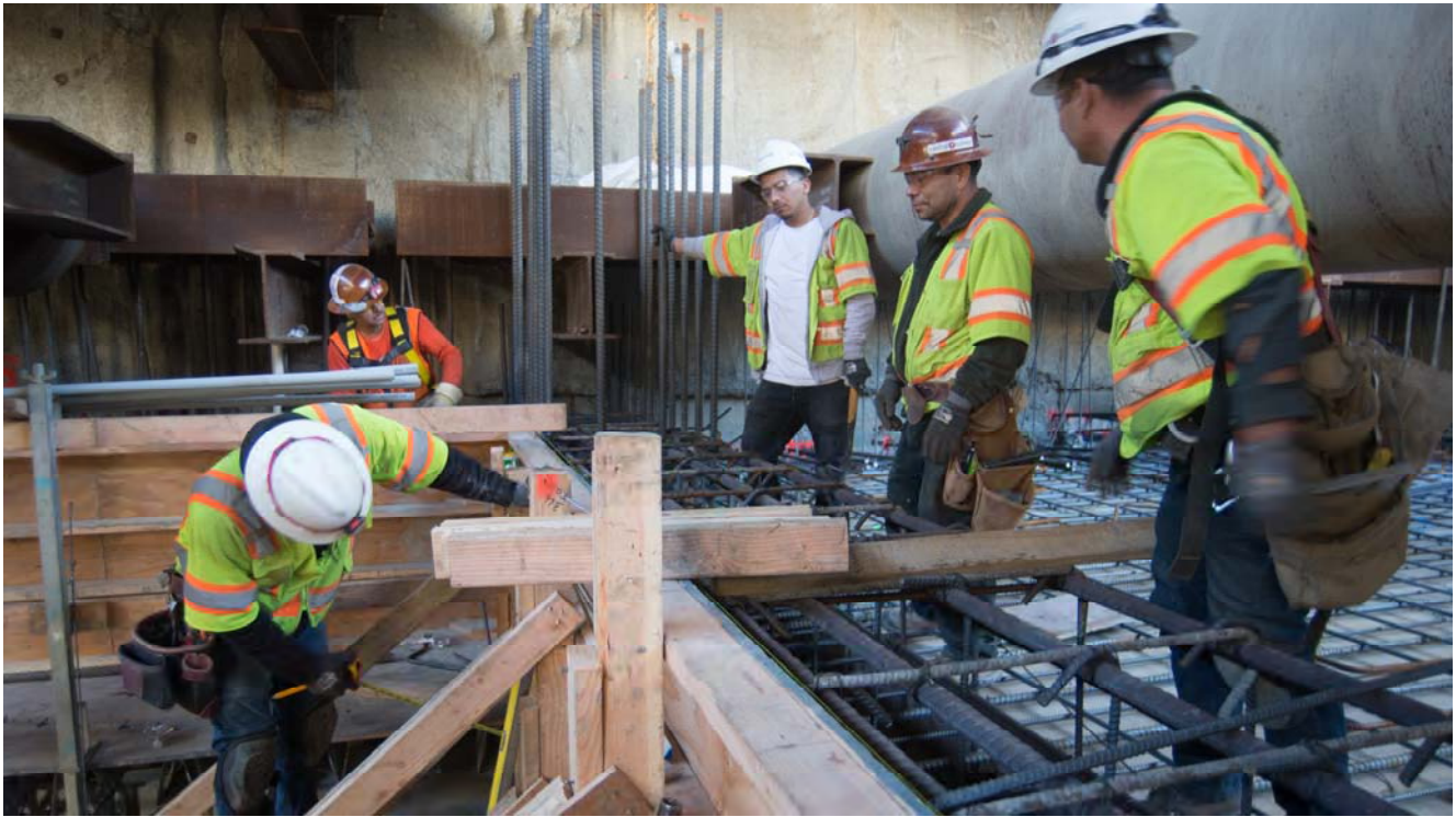
A group of workers install rebar and concrete forms as part of mezzanine floor slab construction on the west side of the station headhouse.
