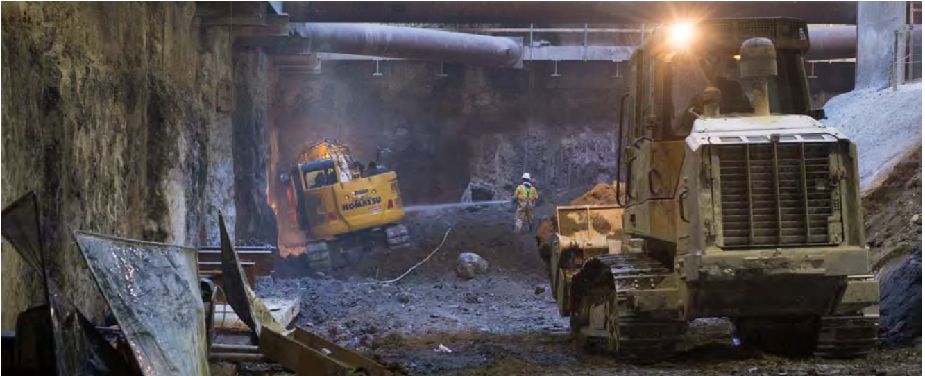
An excavator fitted with a jackhammer removes unneeded concrete from the base of the headhouse slurry walls following the resumption of excavation work, there.
