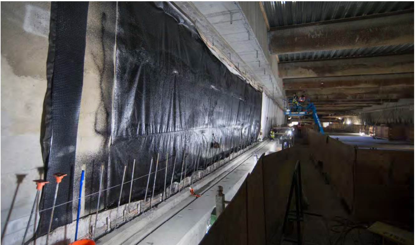
Vinyl sheeting is being installed as part of waterproofing, as seen here on the east wall of the Union Square/Market Street station box.
