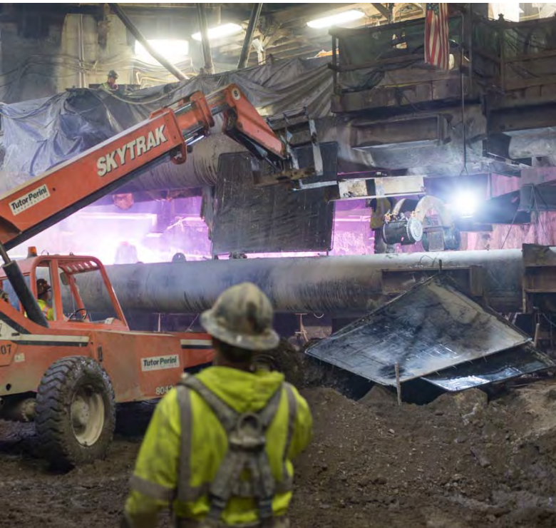
2 Temporary bracing is installed to prepare for the next push of excavation
