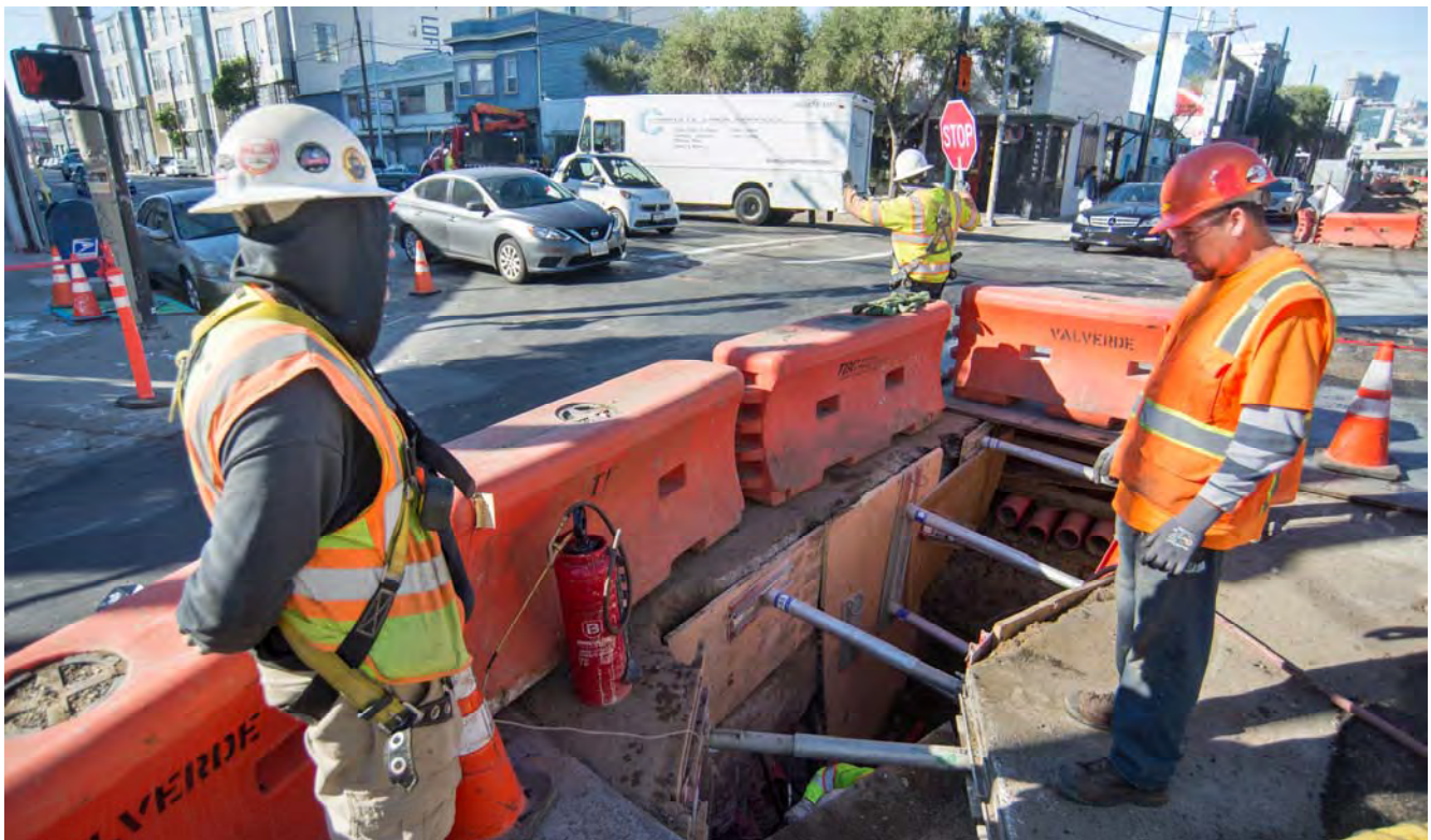
Workers continue installing utility ducts for system signaling and communications, on the south side of the 4th and Brannan intersection.
