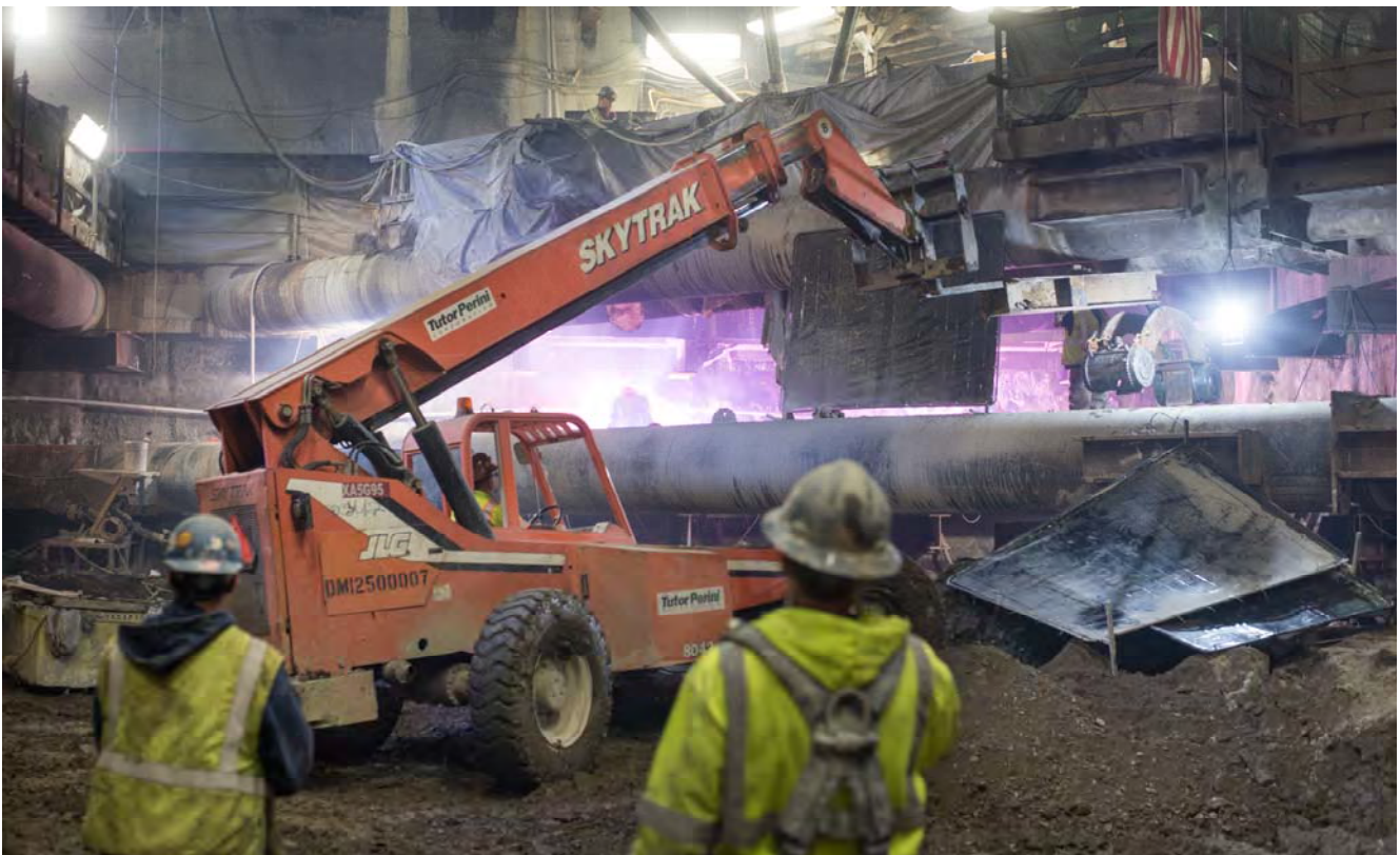
To prepare to resume excavation inside the Chinatown Station headhouse, crews are installing temporary steel reinforcing where they can before digging begins.
