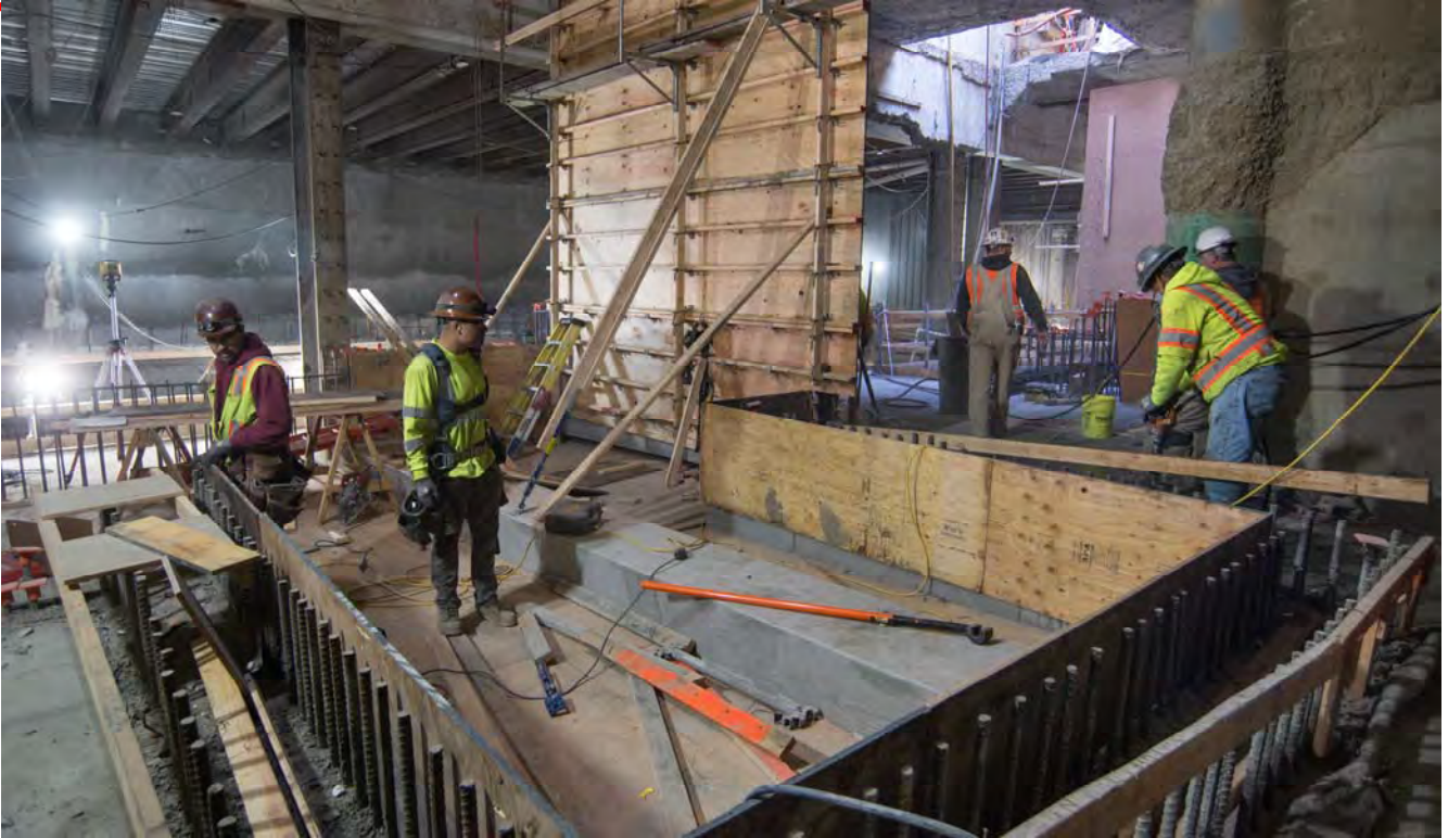
Concrete forms for the north concourse floor slab and some internal walls are being built, shown here where the concourse meets the Union Square Garage structure underground.
