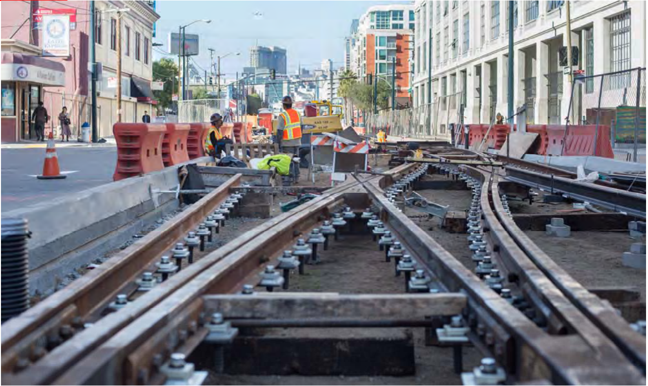
View looking north at the new double track crossover being installed at 4th and Bluxome.
