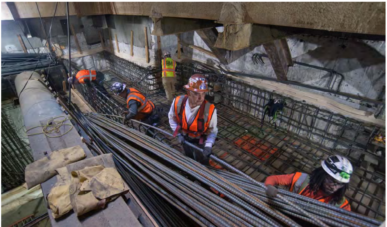
A team of ironworkers places massive lengths of rebar at the north headwall, under the Geary and Stockton intersection.
