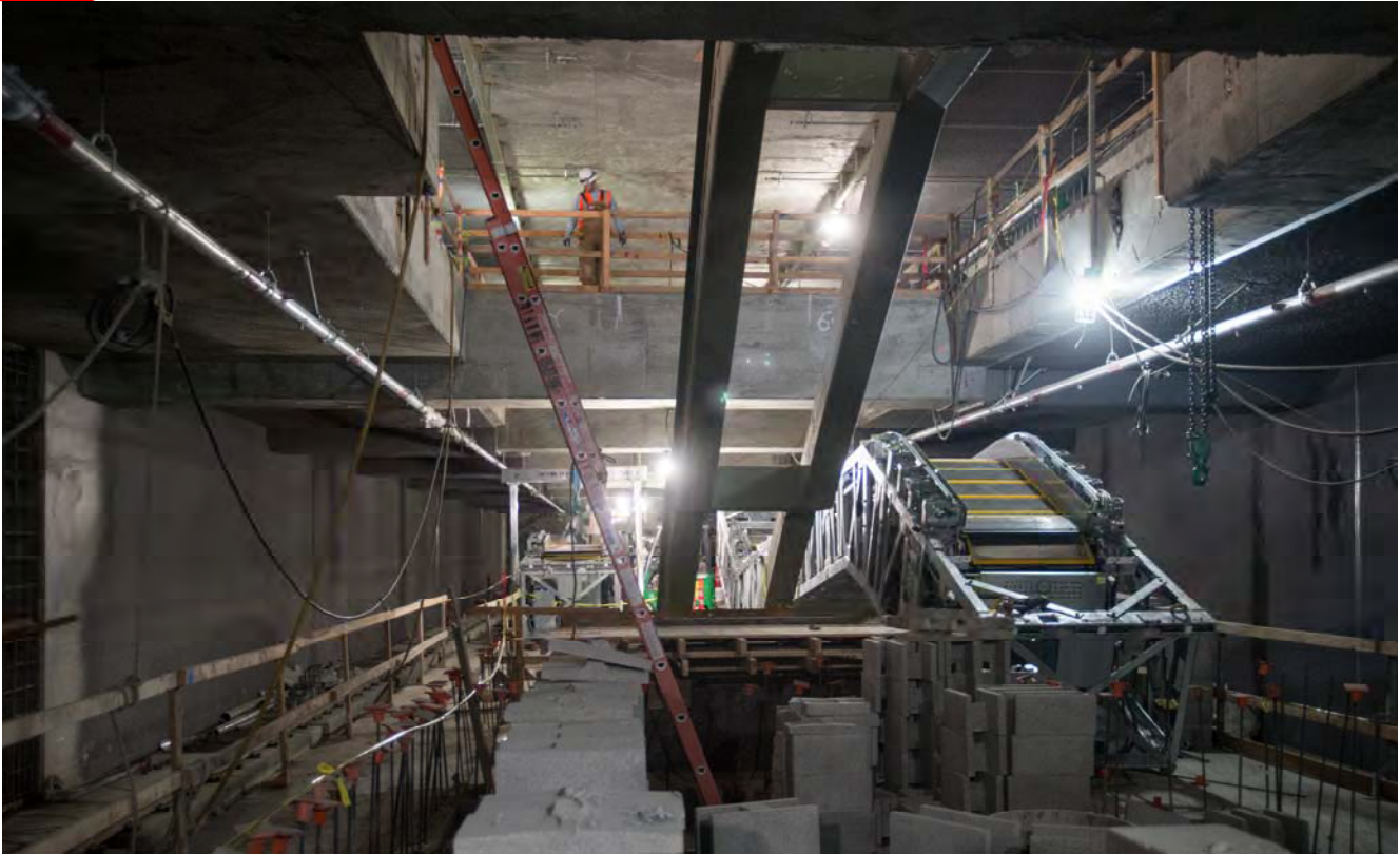
Two escalators slated to be installed at the south end of the Yerba Buena/Moscone Station platform have been lowered into place using a rolling gantry crane.
