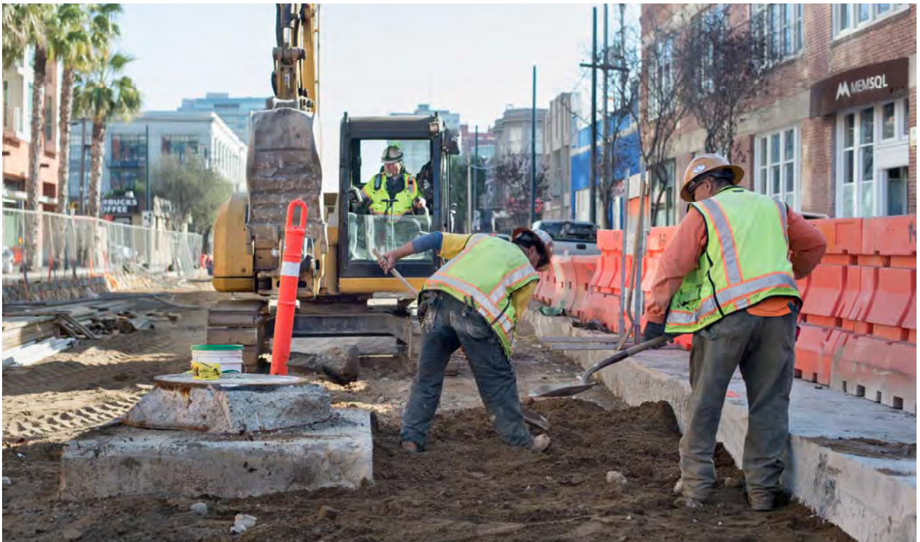
Workers shovel soil to help grade the worksite near a manhole and utility vault at 4th and Welsh.
