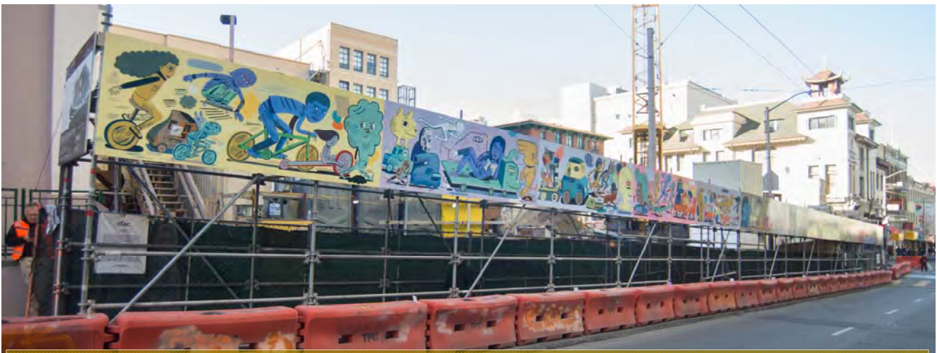
New art has been installed by the SF Arts Commission on the safety scaffolding adjacent to the Chinatown Station worksite.
