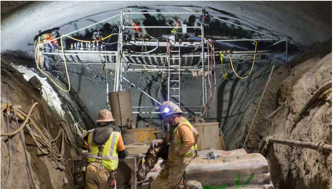
A scaffolding inside the top heading of the south platform cavern's center drift allows workers to get up close to the current face of excavation for soil improvement and shotcrete work.
