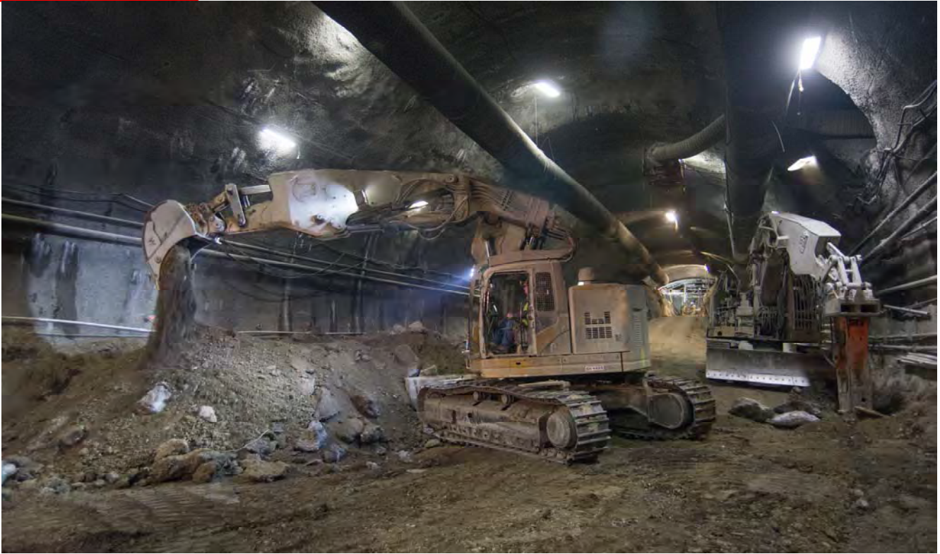
A large excavator collects excavated material inside the southern portion of the station platform cavern prior to removal offsite.
