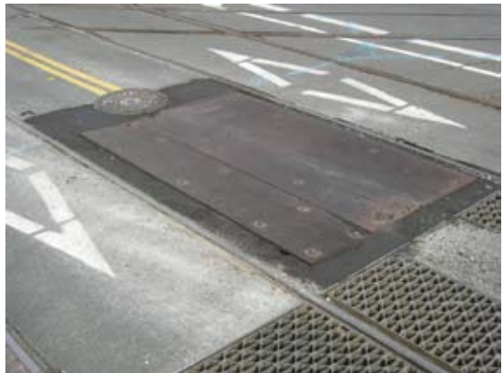
This construction plate lacks required non-skid coating.
